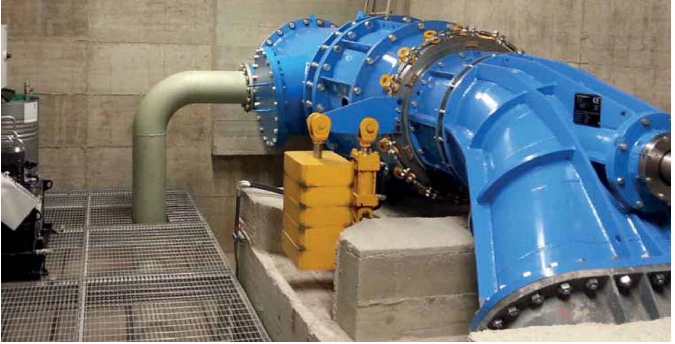
HPP Terni - Italy
