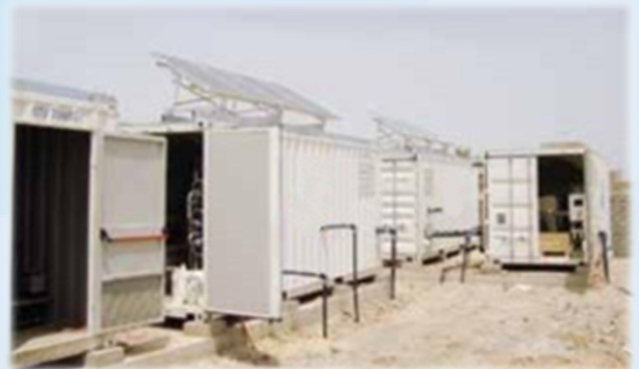
Quartz filtration unit for suspended solids removal.
