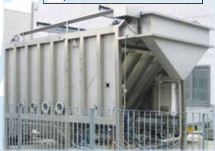
Flotation plant - Q = 1000 m 3 /h
