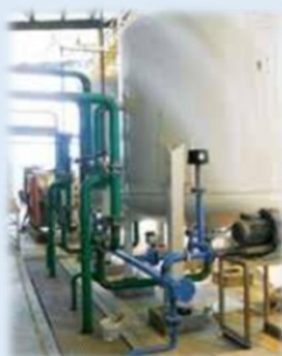
Quartz filtration unit.
