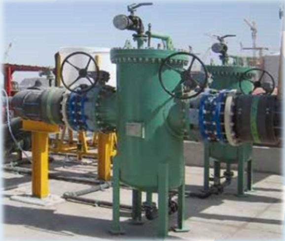
View of filtration system with valves.
