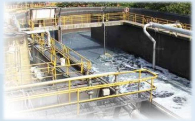
Wastewater treatment by 100% biological technology.
