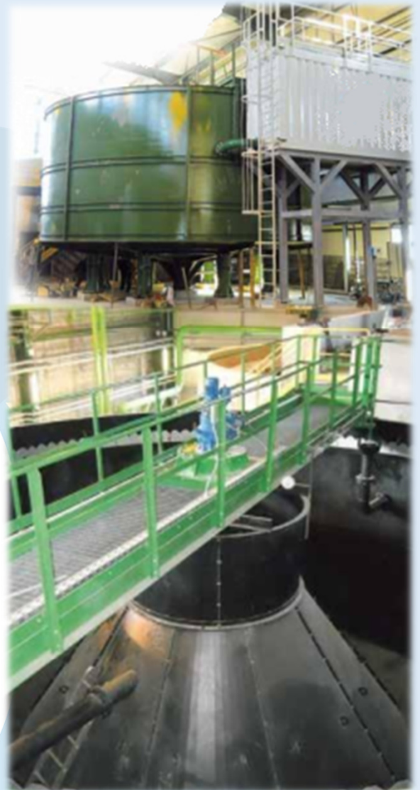
Steel sedimentation tank for mining industry.
