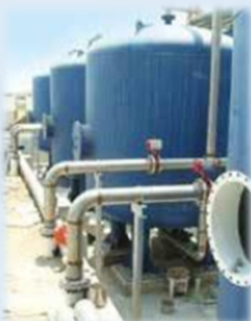
View of sand filtration.
