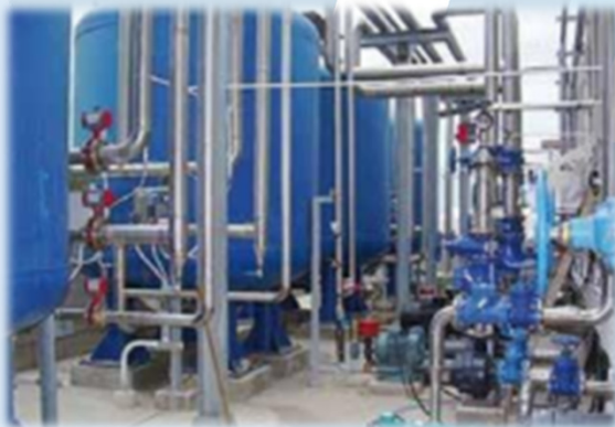
Quartz filtration unit for suspended solids removal.
