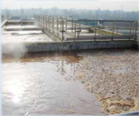
Oxidation tanks - Q = 1500 m 3 /day.
